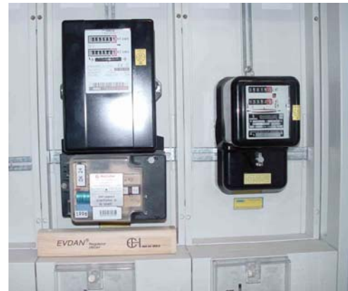
House regulator installed on fuse box
